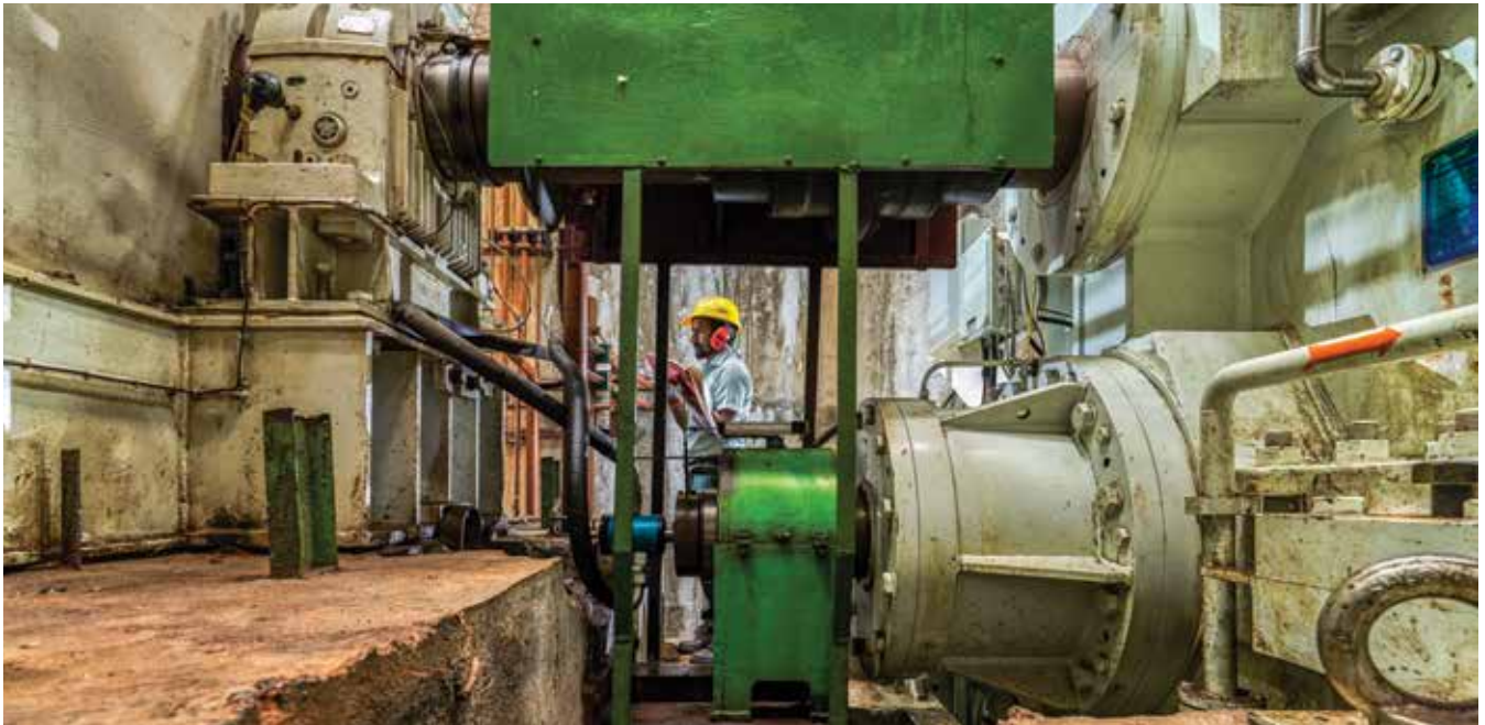
AMR Power Pvt. Ltd., Karnataka
